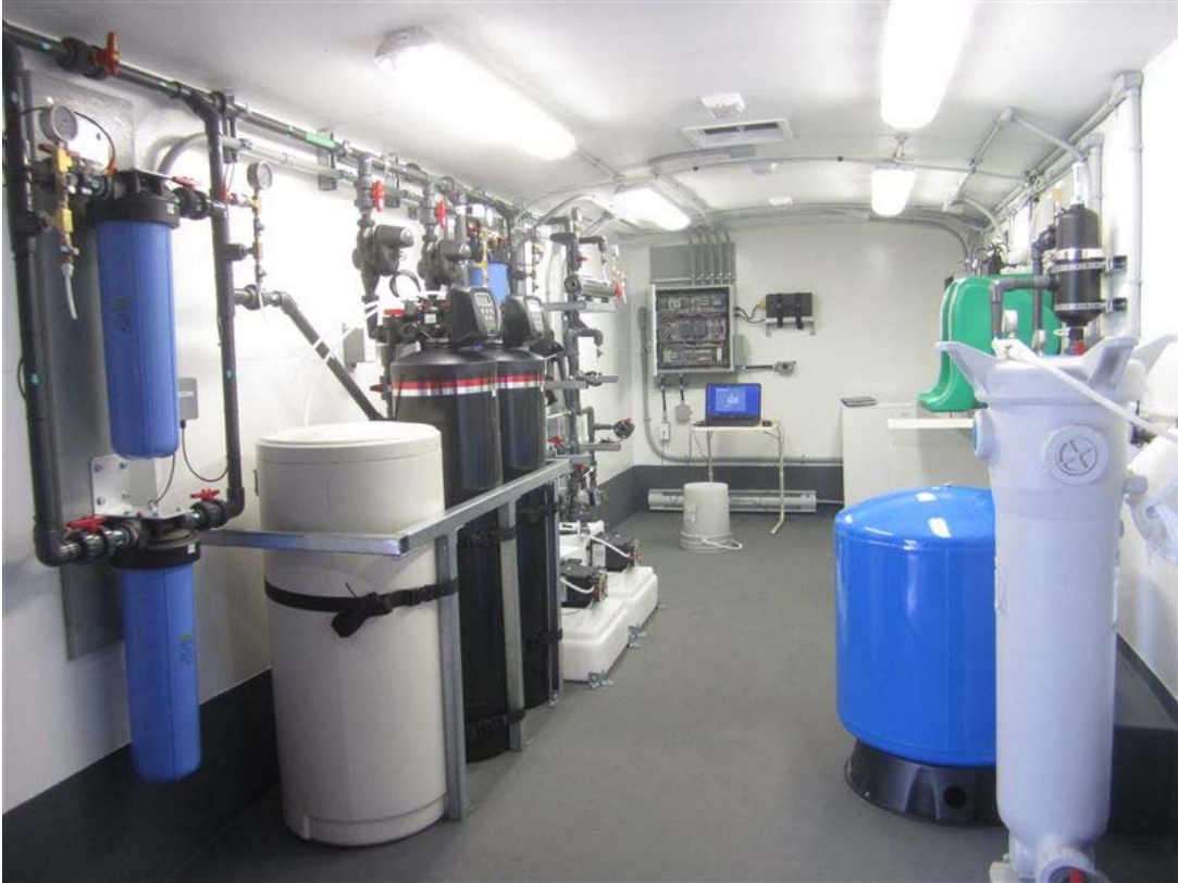
The interior of the new treatment plant.
